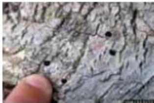
1/8-inch D-shaped exit holes created as EAB beetles emerge
